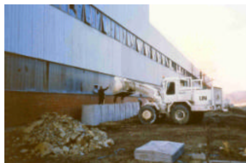
Figure 39. This piece of armoured plant is being used to build fortifications for a UN peacekeeping unit in Bosnia. However, the main use of such equipment in a humanitarian demining context is rubble removal in built up areas (photo by the author, 1994).
