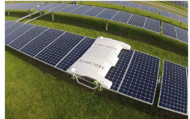
Figure 13.1.3 Solar tracking system with robotic cleaning
