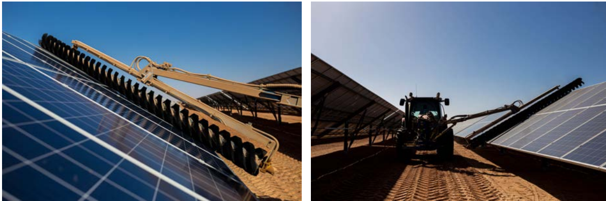
Benban 150 MW plant, Aswan Egypt
