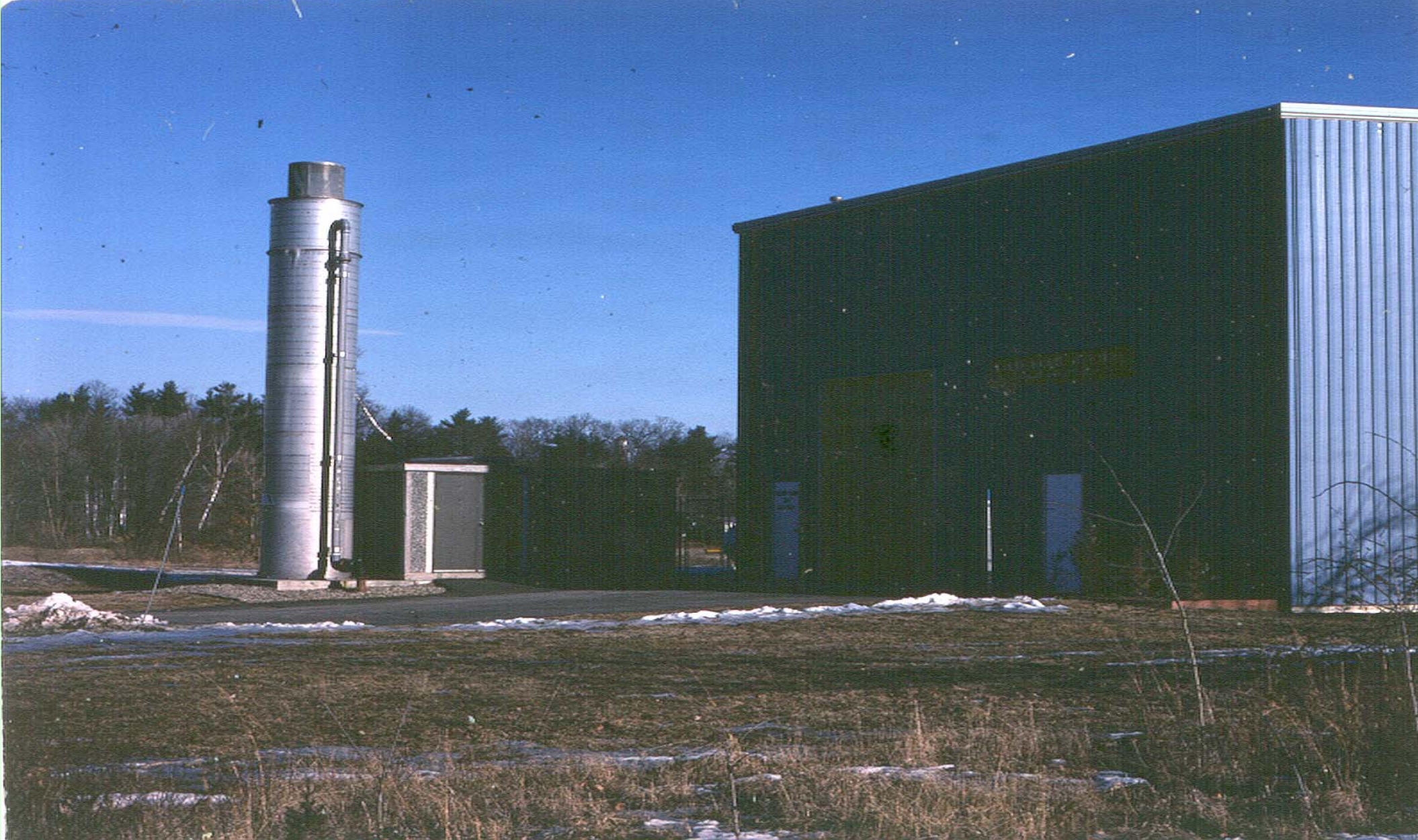
Air stripper in Acton, MA. It is installed on an Acton public supply well affected by the W.R. Grace Superfund Site. Image courtesy of Peter Shanahan.
