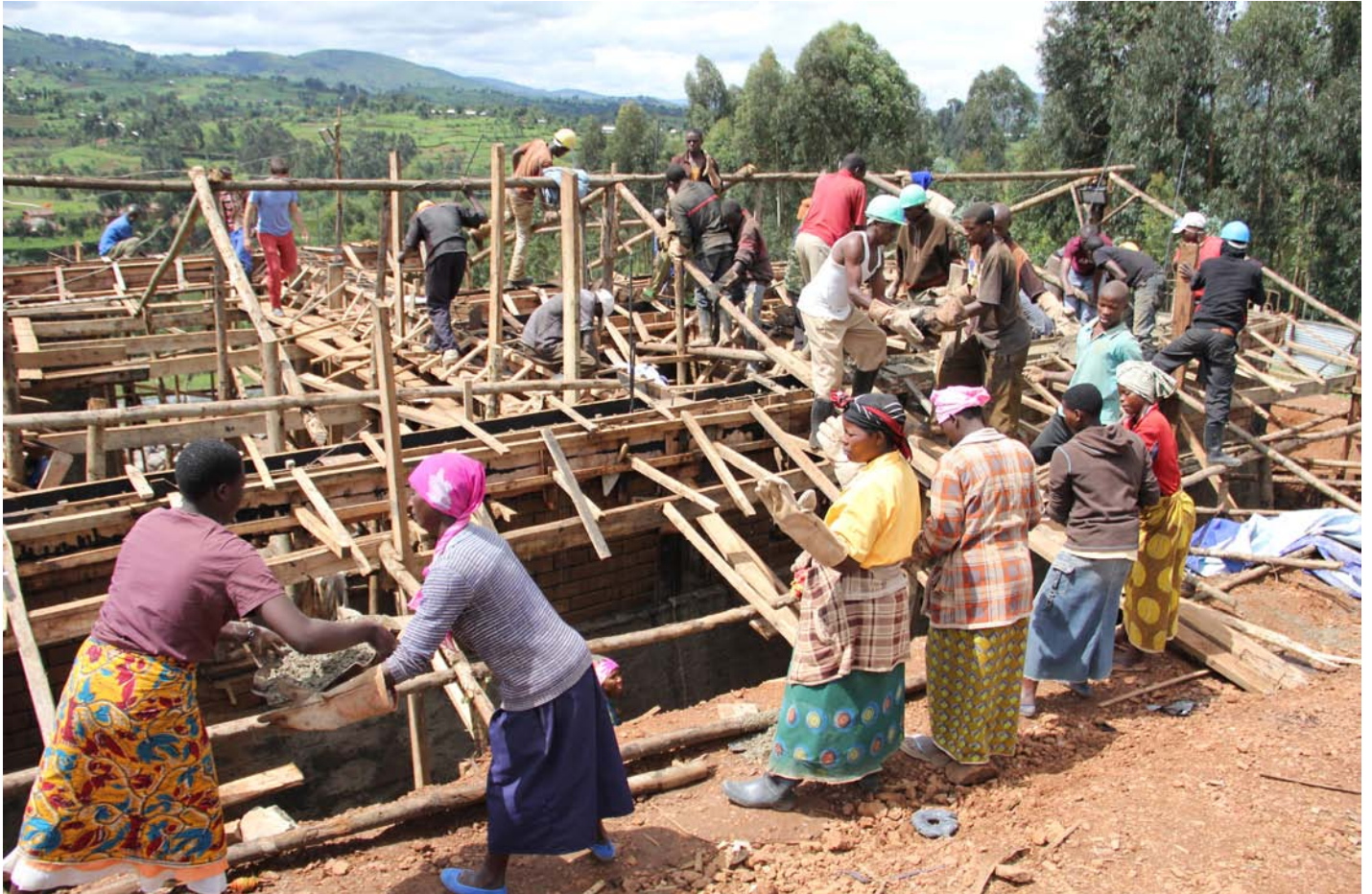
Public interest design practices were found, by the Latrobe Prize research team, to not only address a community's immediate needs, but often build the assets and capacities of that community. Worksite at Butaro Hospital Doctor's Housing, MASS Design Group.
