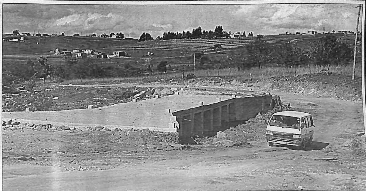
A kombi passing next to the newly constructed bridge where 14 people died after the Quantum they were in was swept away by floods two years ago at Lushikishini. The deadly bridge was at the level in which the kombi is passing at, although this is not to suggest this is the one that drowned with the people. (Pics: Mloni Mpanza)
