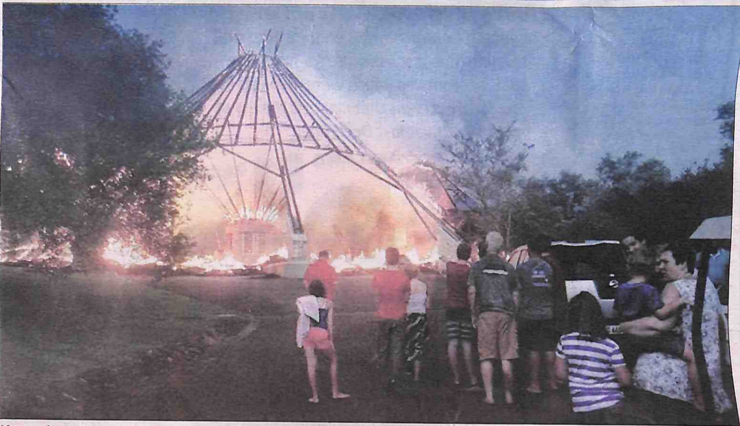
Yesterday's thunderstorm left a trail of destruction after lightning struck the Nkonyeni Golf Estate gate house, igniting the thatched roof, razing it to the ground. (Courtesy pic)
