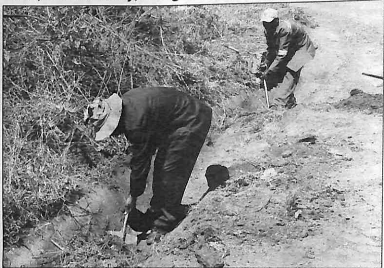
COME RAIN OR SUNSHINE: Municipal Council of Manzini employees hard at work unblocking storm water drains along Logwaja Street in Extension 6.
