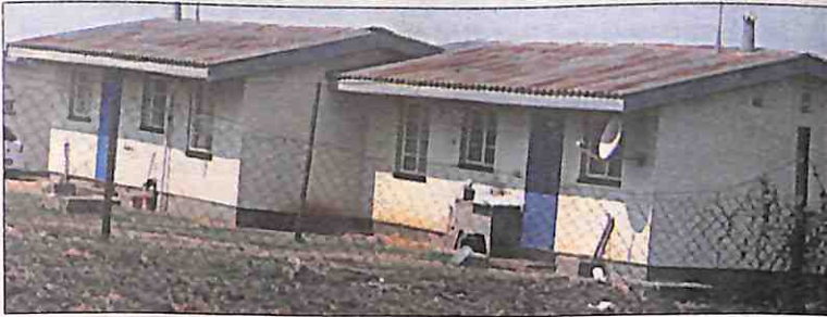
DILAPIDATED: Some of the old police houses which had been vacated by some senior police officials based at Sigodwveni police station.
