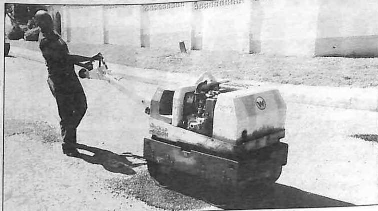
COATES VALLEY: An employee of the Municipal Council of Manzini busy patching potholes in Acacia Road, Coates Valley, using a compactor.
