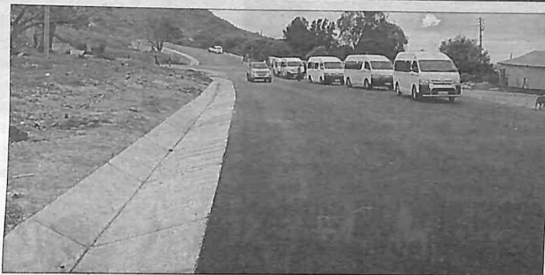
Motorists have commended the new look section of the nearly completed MR3 road between Matsapha and Manzini. (Pic: Thembeke Dlamini)
