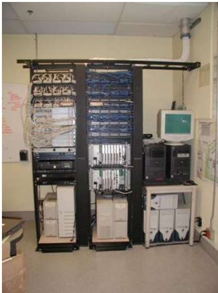
Figure 1-5. RDCC private data center (courtesy of Microsoft)
