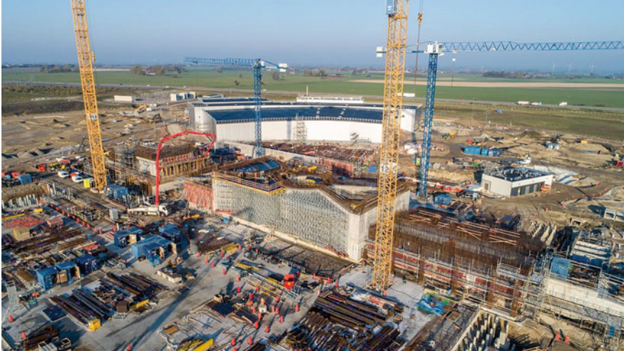
Fig. 1 ESS under construction in Lund, Sweden. The central concrete structure will house the neutron production target
