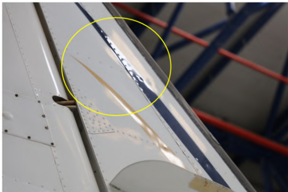
Figure 2. The gaps could be due to lose fasteners in edge of skin lap. Defect can easily be missed if not inspected standing on a work stand. The light plays an important role in damage detection. Photo taken at Abu Dhabi Polytechnic Hangar.
