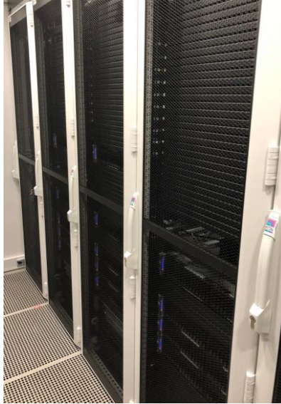
Figure 4. HPC cabinets with servers and nodes.
