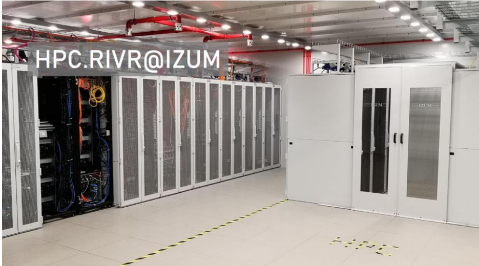
Figure 6. The equipment and dedicated space for HPC-RIVR.
