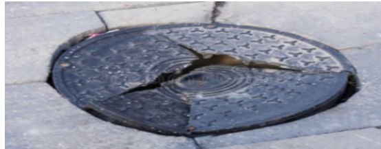
Figure 1. A damaged manhole cover
