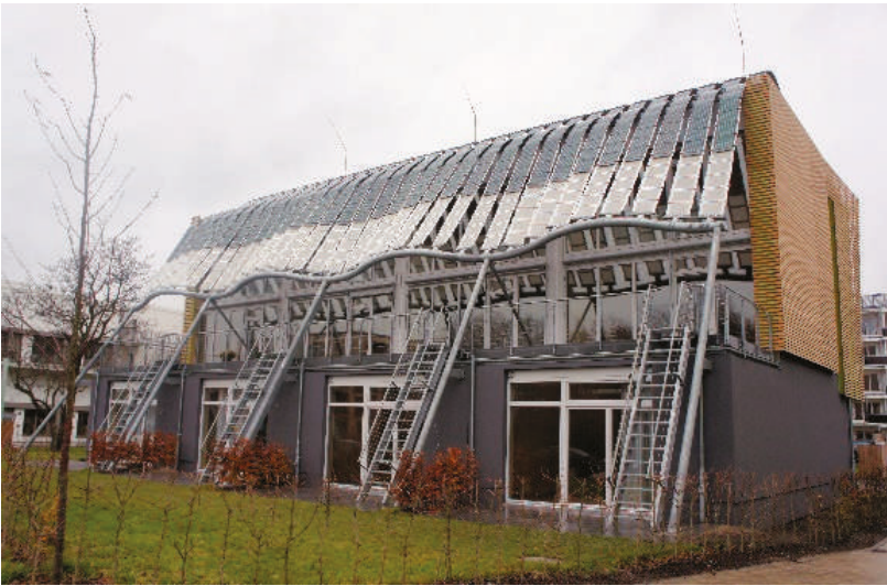
Figure 11. Solar electricity generating thin-film system independent of the building (photo by W. Celadyn).
