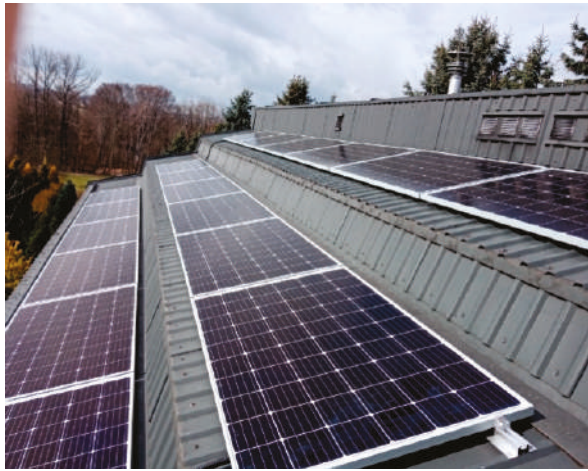
Figure 8. Stepped roof with PV monocrystalline photovoltaic panels installed at the recommended angle of 15°. Location: 49°57' N, 19°55' E (photo by W. Celadyn).
