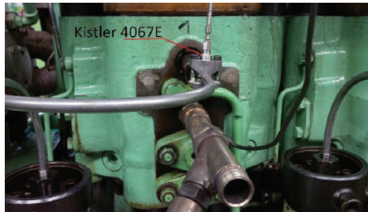
Figure 1. Installation of the Kistler 4067E injection pressure sensor (in the background, the electric cable of the Kistler 6353A24 combustion pressure sensor protruding from the indicator cock).
